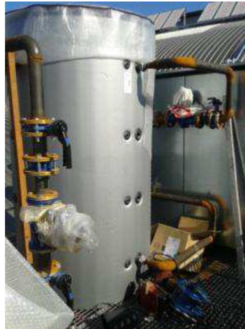
Buffer tank, 2 m 3
