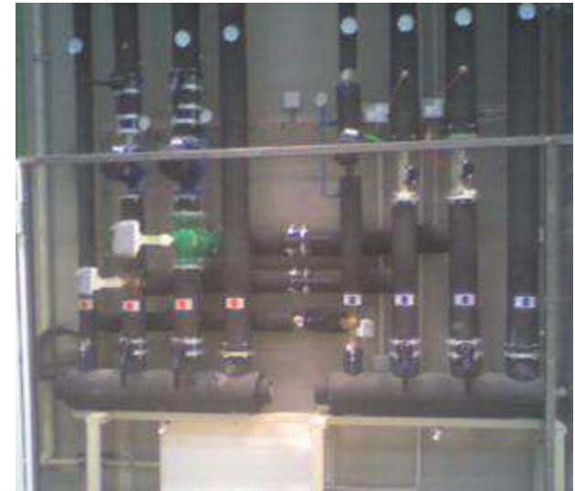
Secondary circuit, hydraulic collectors
